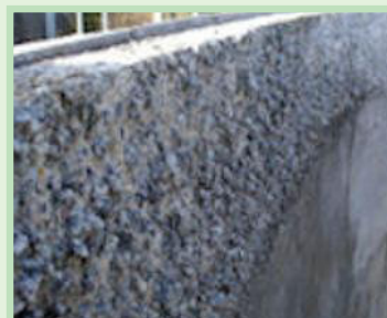
Figure 4: Inside view of a concrete digester after operation
