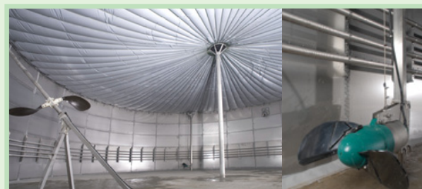
Figure 8: Inside view of a stainless steel digester tank 7
