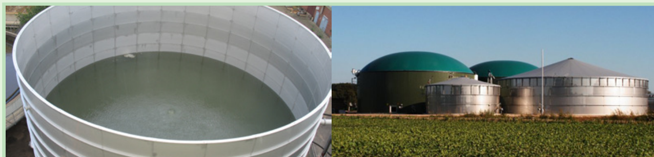
Figure 7: Interior view of stainless steel storage tank (left) and exterior view of storage and digester tanks 6
